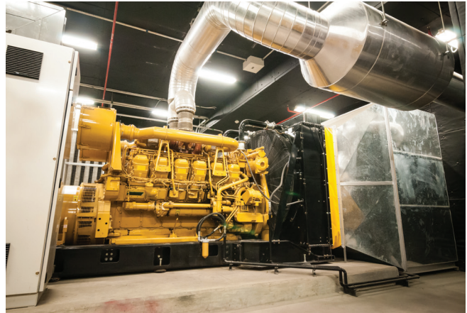
Diesel power generators are used by many research facilities for backup power of vital ULT storage and other equipment in the event of a power outage.
